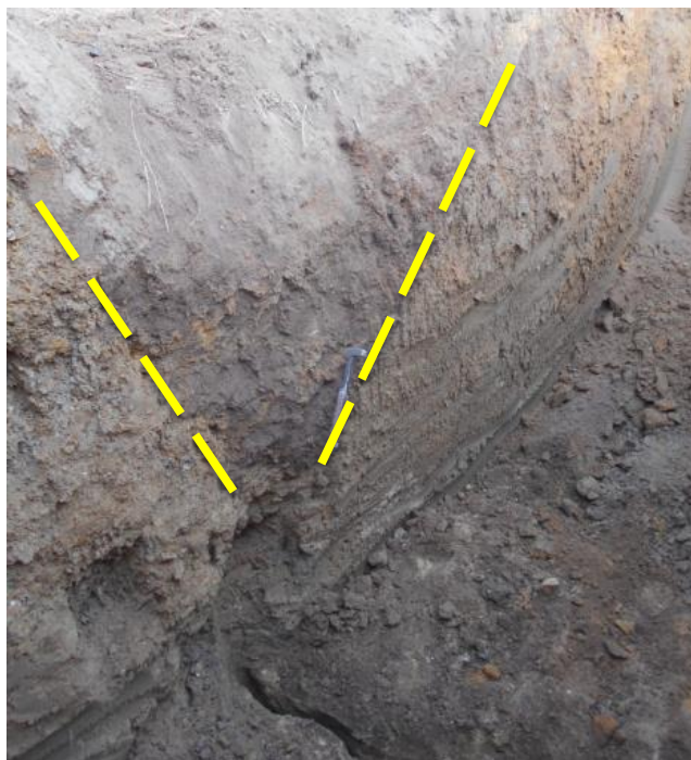
Figure 3-13: V-shaped zone in TP03 above the collapsed tunnel and crack in the rock below.
