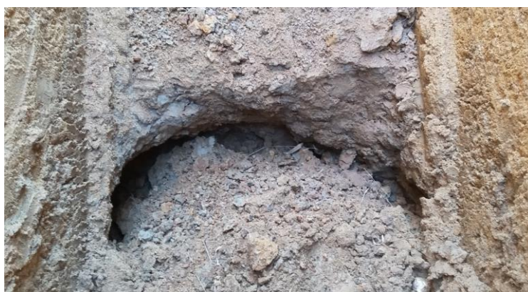
Figure 3-14: View downwards into TP18 showing the subterranean tunnel running from right to left.
