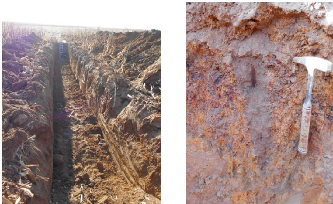
Figure 3-17: Trench in Area 2 at TP10 and hillwash infilled crack in the residual sandstone.
