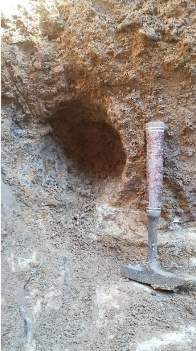
Loose material of collapsed sub-terranean tunnel excavated at bottom of TP18 above infilled crack in rock.
