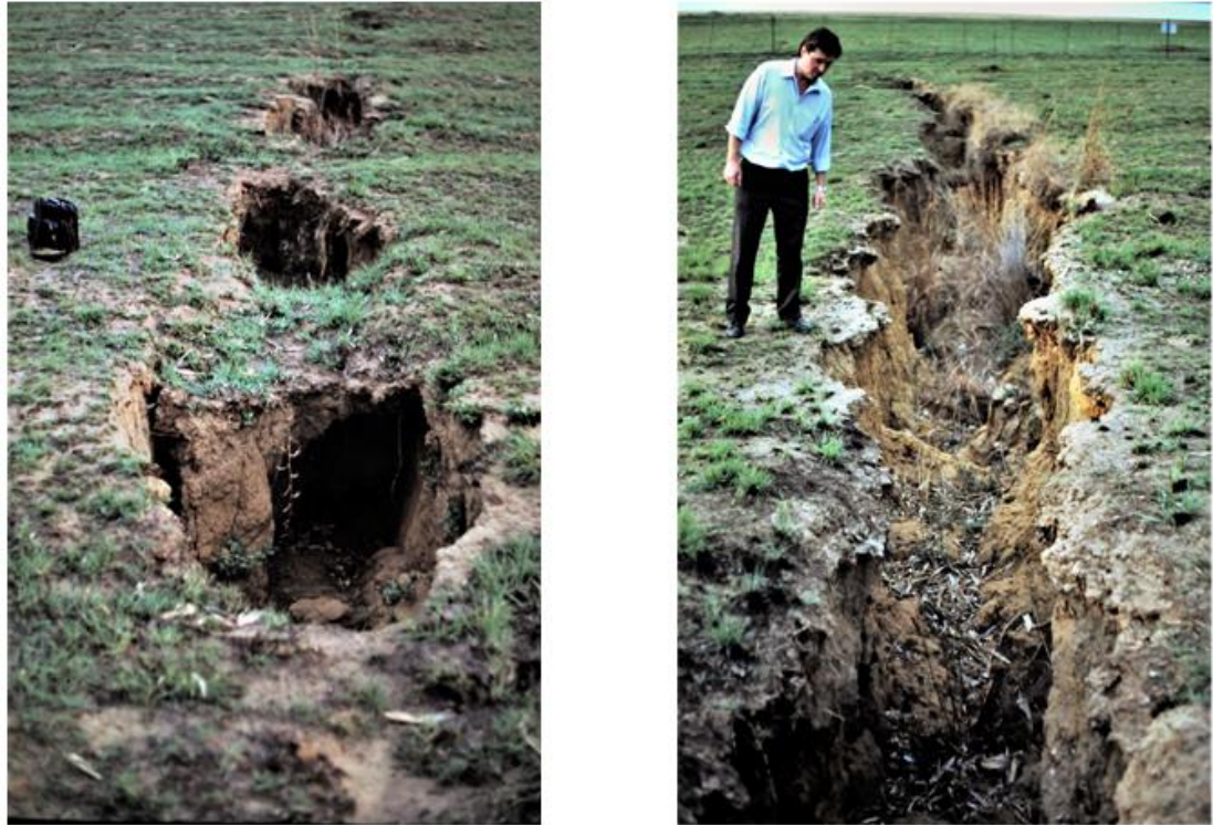
Figure 2-13: Progressive failure of the cover to the subterranean cavity (Van der Merwe, 2018).
