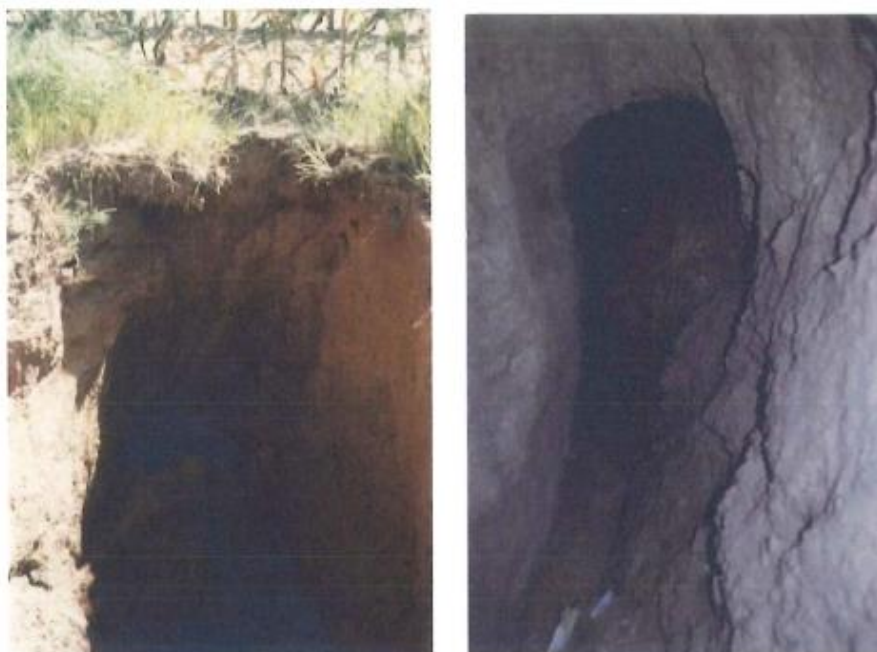
Figure 2-2: Photo of the first sinkhole at Sigma Colliery (left) and subterranean tunnel (right) (Van der Merwe, 1990)
