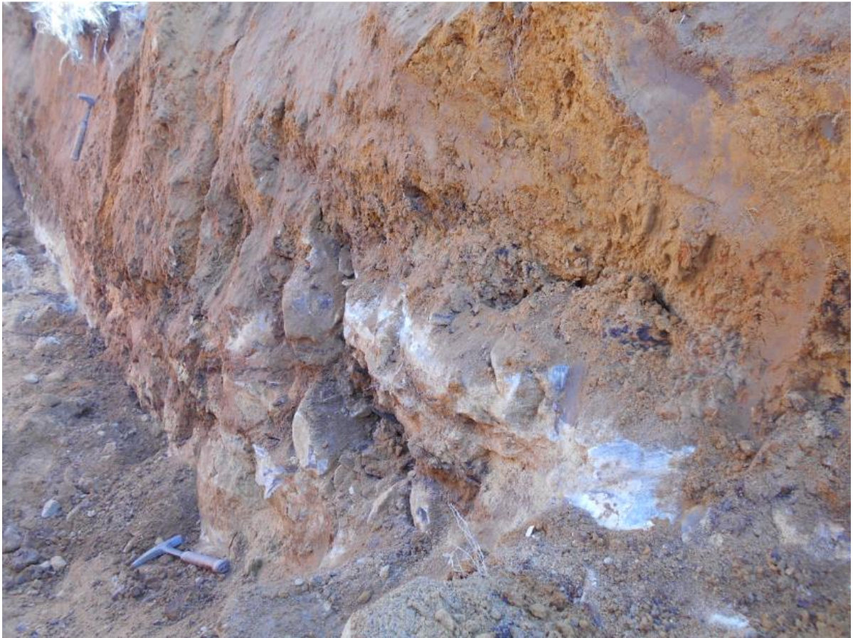
Vertical displacement across fracture zone at edge of subsided area exposed in TP11.
