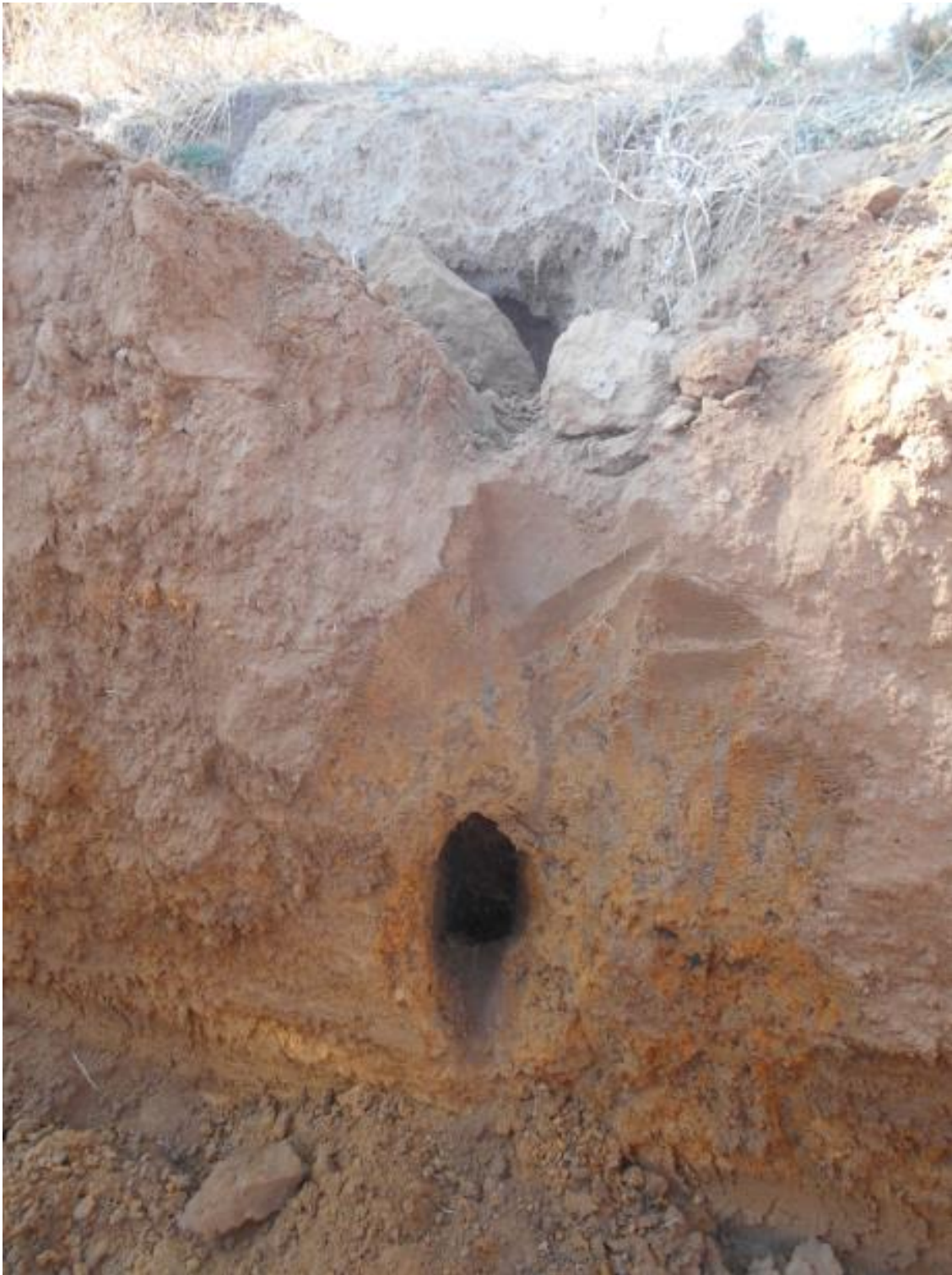
Start of the excavation at TP06, showing the sinkhole on surface and the intersected subterranean tunnel below.
