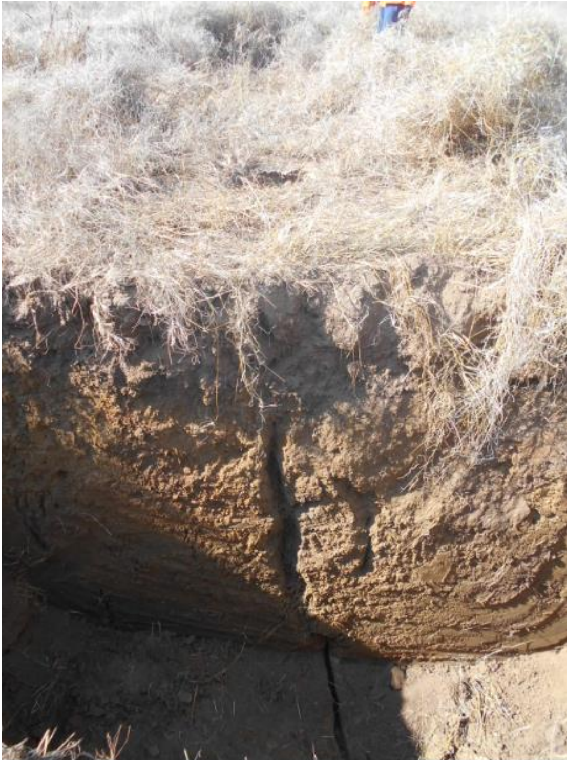
Looking east at TP01, with sinkholes at TP02 and TP03 in the background.
