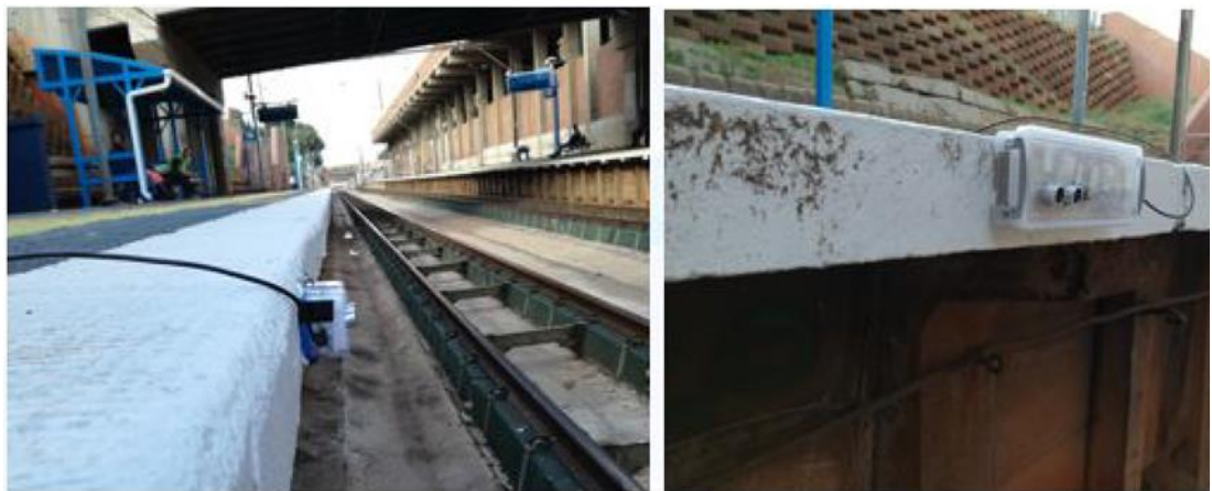
Figure 3-14: Prototypes mounted on the platform to measure the horizontal gap size between the train and the platform
