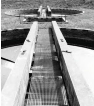
Settling tanks covered in algae (Renton, 2018)
