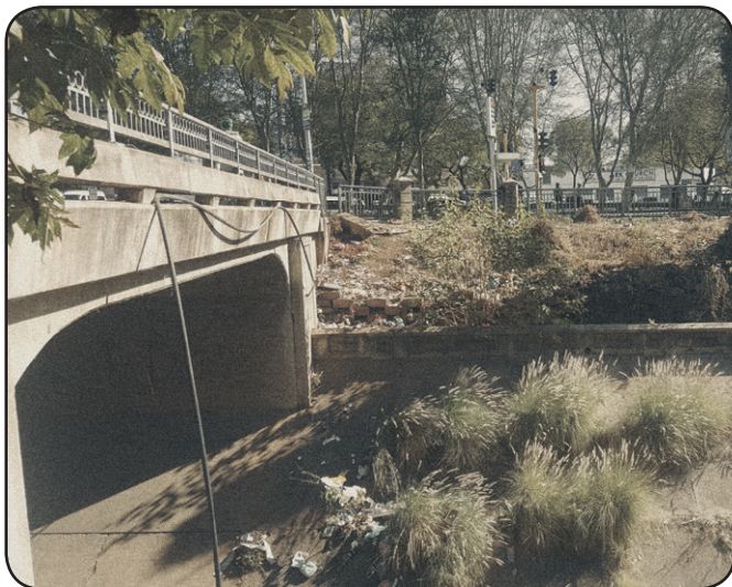
Figure 3.37: Degraded river bank (Author 2019)
