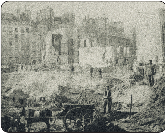
Figure 1.2: Demolition of Butte des moulins for Avenue de l'Opera (Desconicido 1870, edited by Author)
