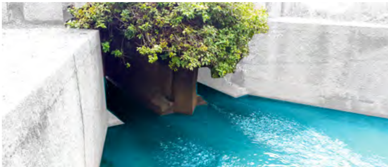
Figure 30: Damaged River System - Nooitgedag Spruit
