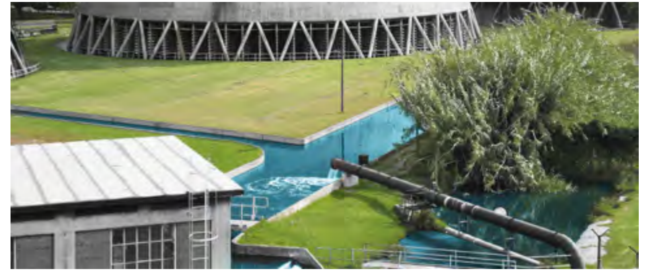
Figure 32: Water Supply to Cooling Towers
