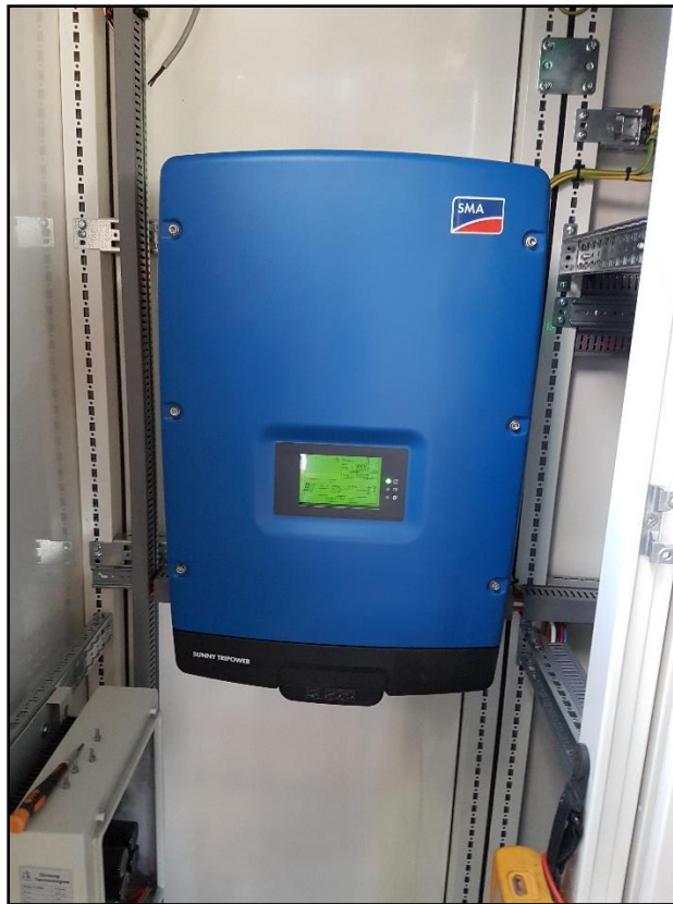
Figure D-13: Inverter
