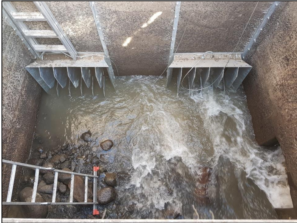
Figure D-5: Inlet shrouds in place (upstream side of the scouring section of the intake structure)
