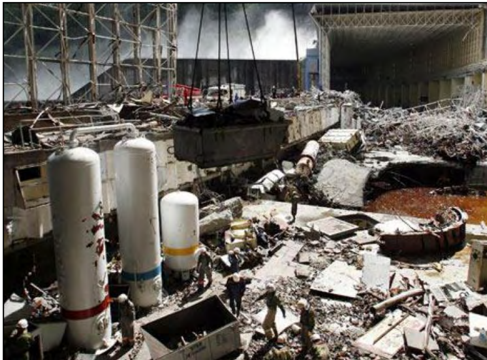
Figure 2-40: Sayano-Shushenskaya Hydropower Plant Flood Damage (Hasler, 2010).
