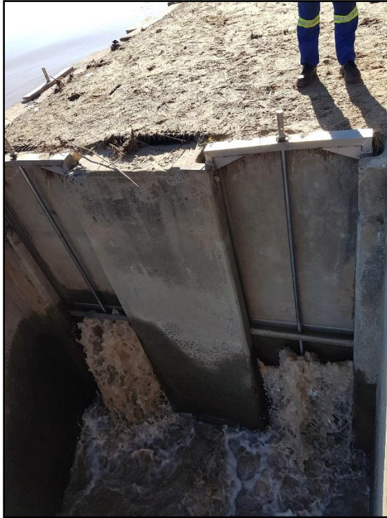
Figure D-1: Scouring section of the Intake structure where the new turbine will be installed
