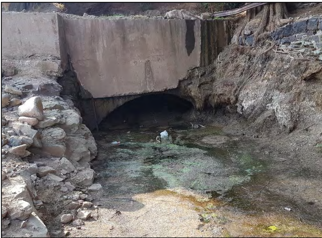
Figure 5-15: Blocked Outlet Structure
