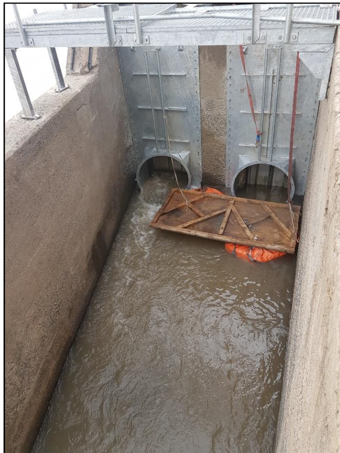
Figure D-6: Face plates in position
