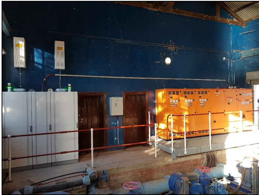
Figure D-11: Powerhouse containing the new control panel as well as the existing control panels for the pumps
