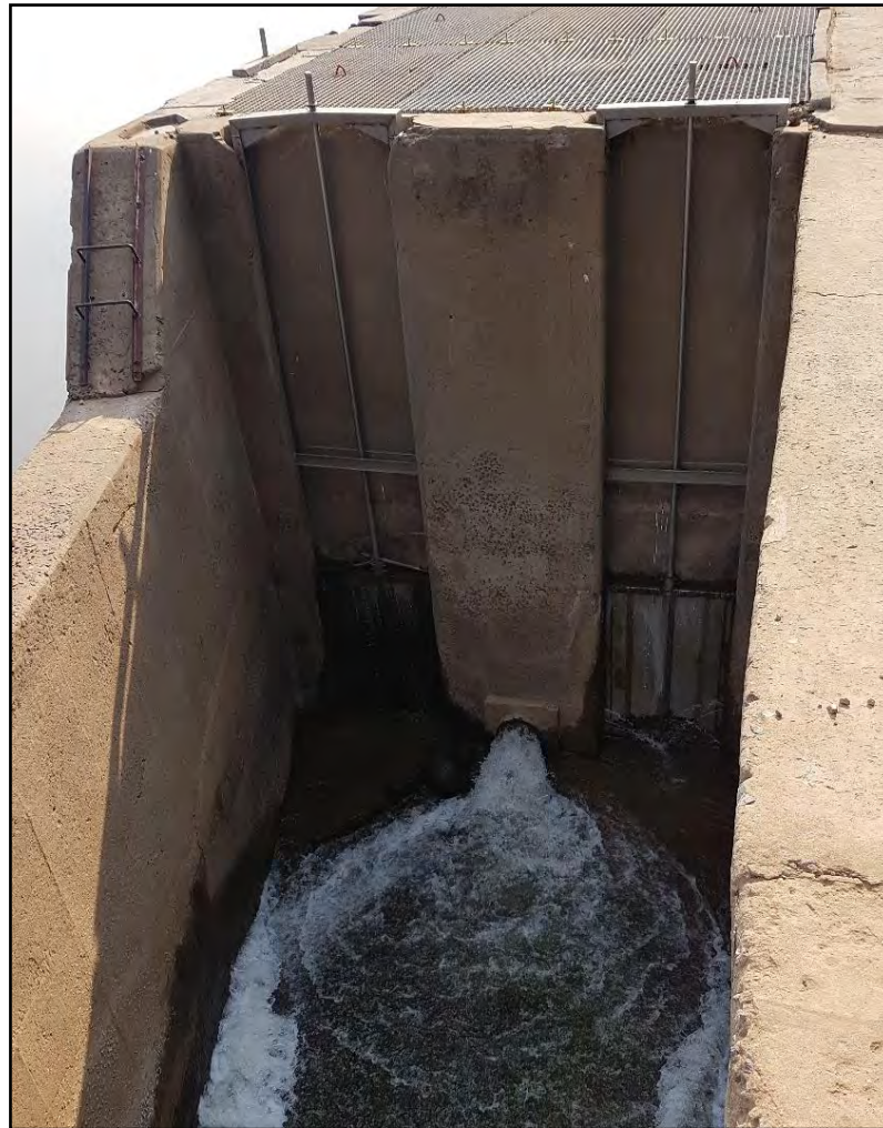
Figure 5-16: Scouring Section of the Intake Structure
