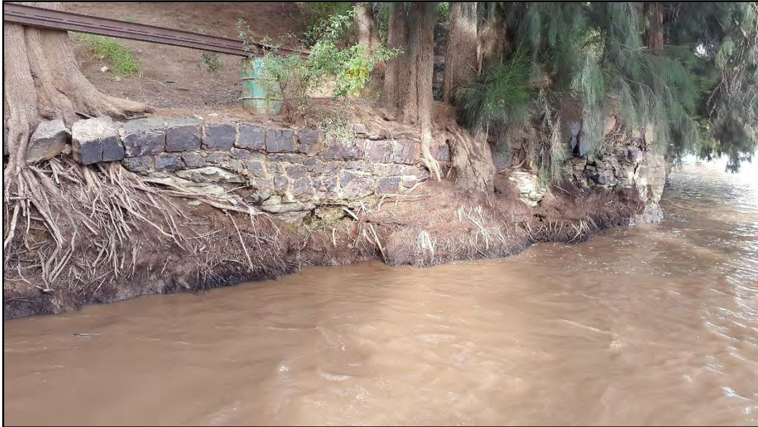
Figure 5-9: Erosion of the River Banks at the Outlet Structure
