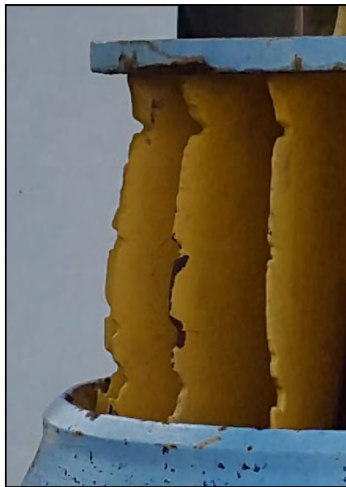
Figure 5-8: Damage on the Runners
