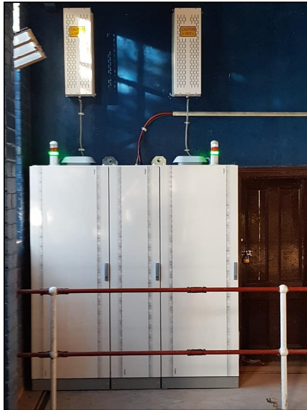
Figure D-12: Control Panel housing the Inverter, Rectifier and Dump Loads
