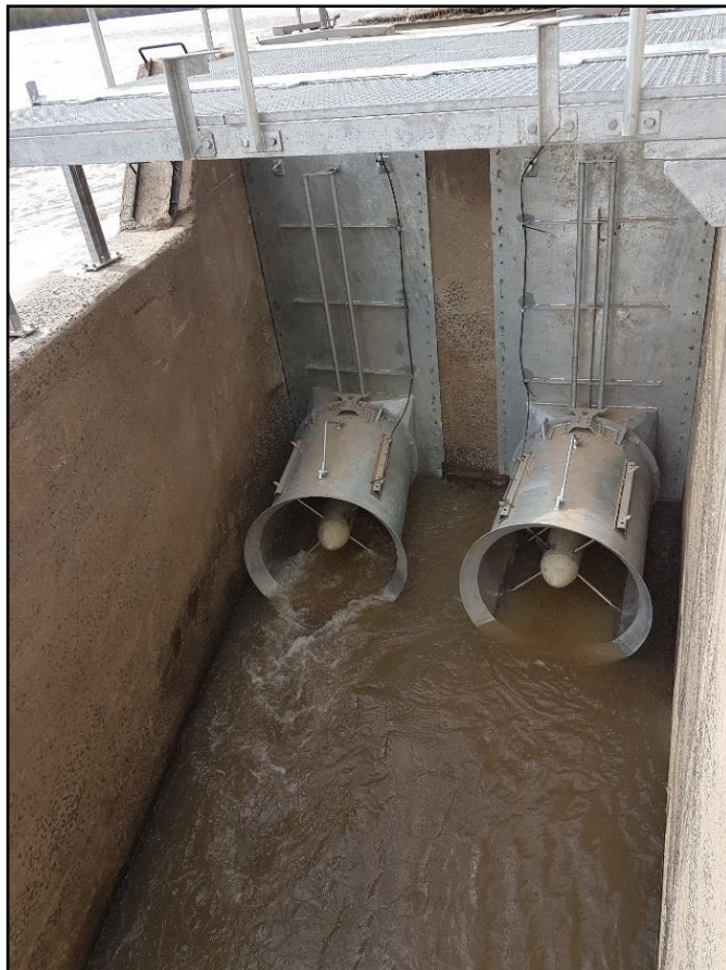
Figure D-8: Kinetic turbines connected onto face plates
