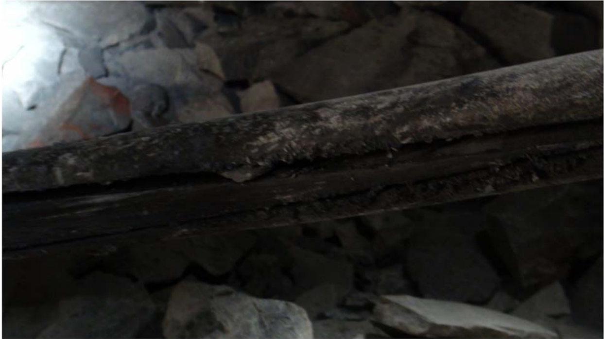
Figure 41: Small rock fragment wedged between the feather and the centre wedge (Author, 2013)
