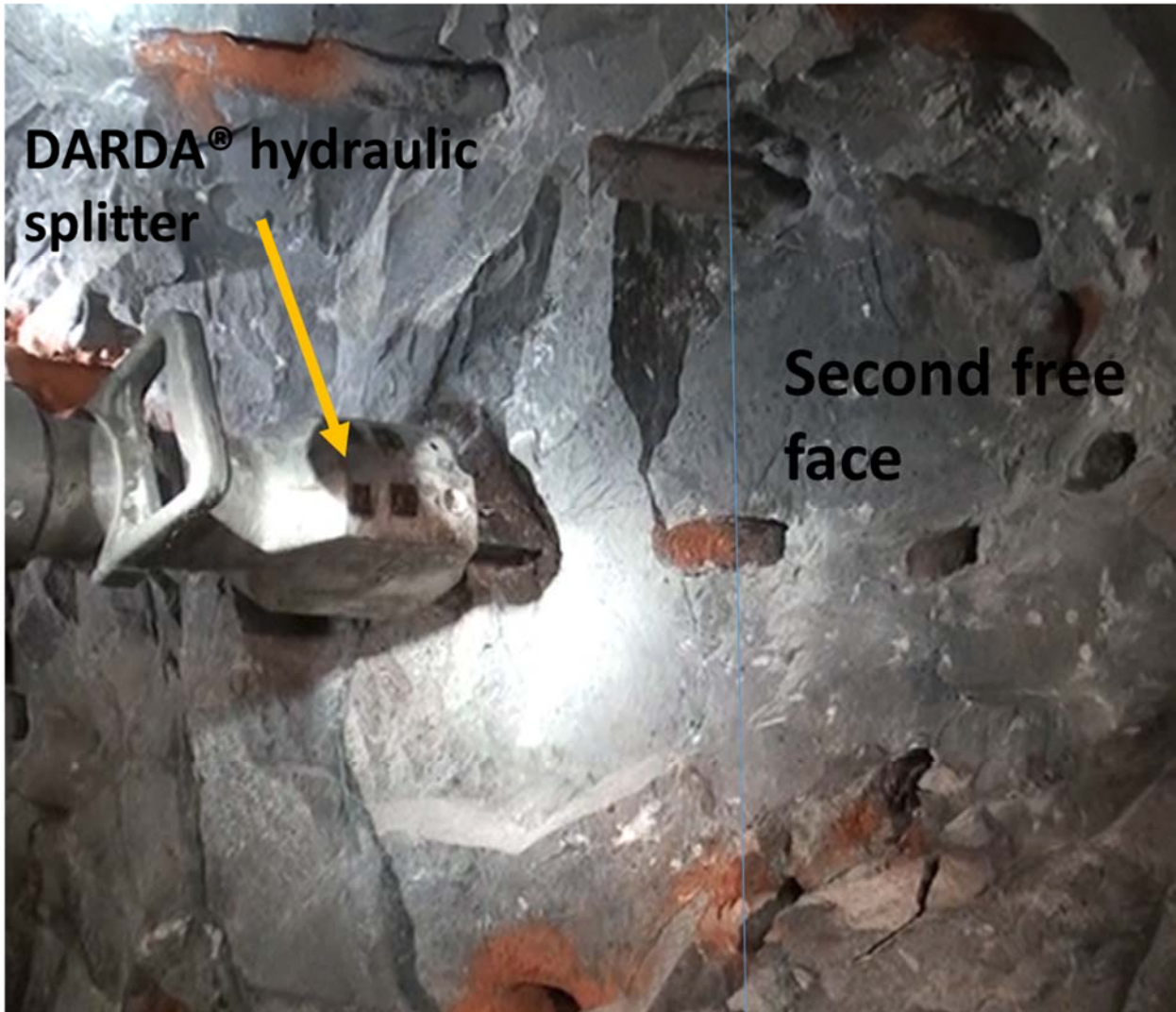
Figure 35: Free face slicing with visible drill barrels parallel to the free face (Author, 2013)
