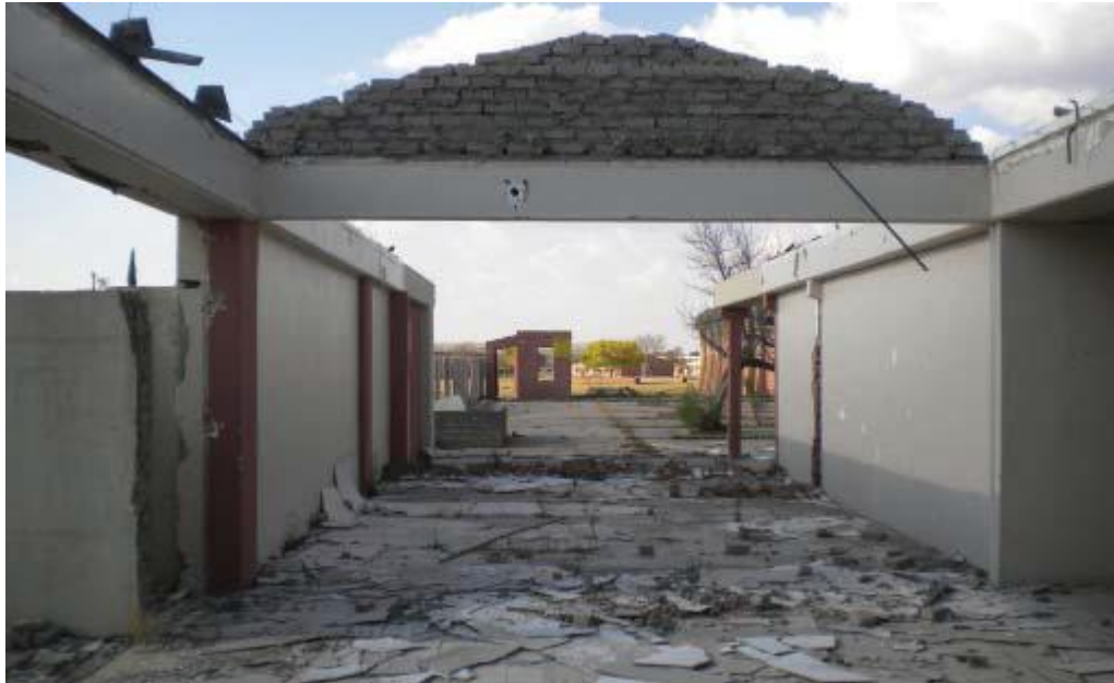
Figure 32: The Merriespruit 3 hostel before the conversion into rental units started Source: Infrastructure News, 2013
