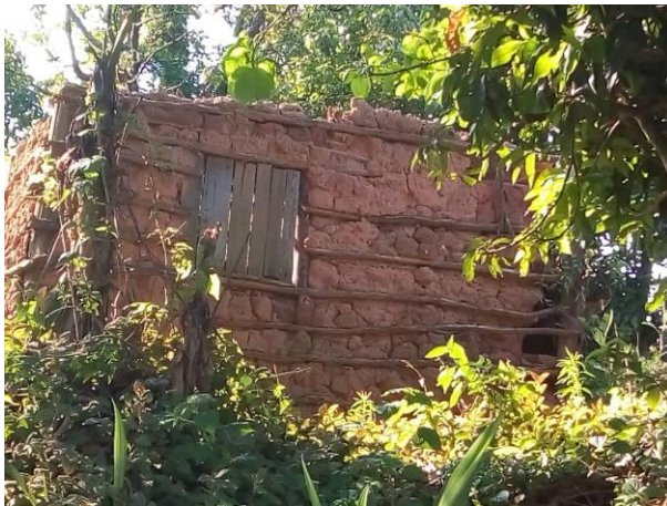
Figure 5.4. Remains of a demolished house at Msunduza
