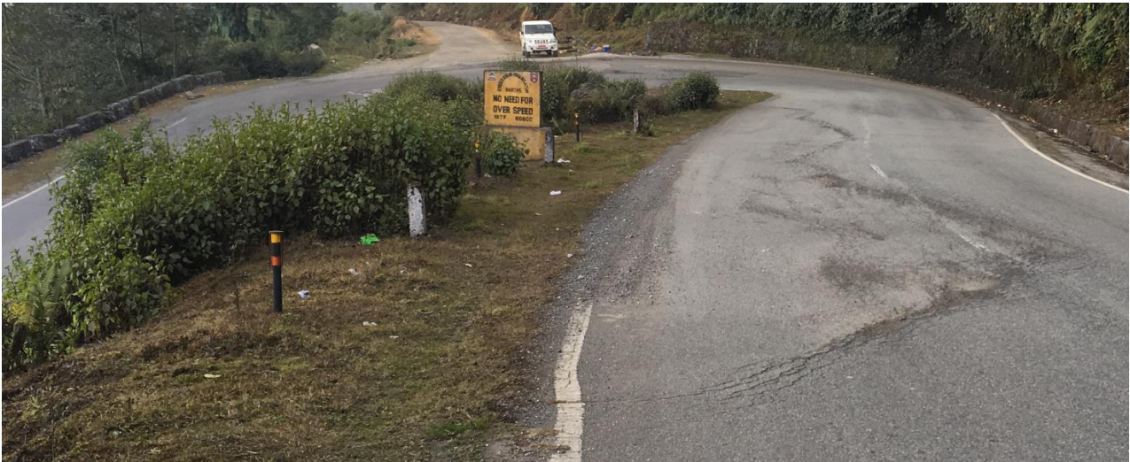
Figure 1 Incipient failure of fill slope made apparent by deformation arcs in asphalt road surfacing
