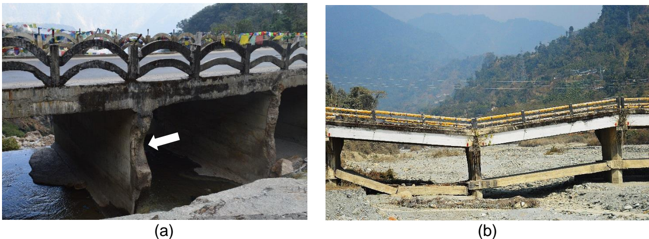
Figure 4 Examples of damage to bridge causes by high energy flows: (a) impact of boulder on culvert (see arrow); (b) the results of scour, seen in the dry season
