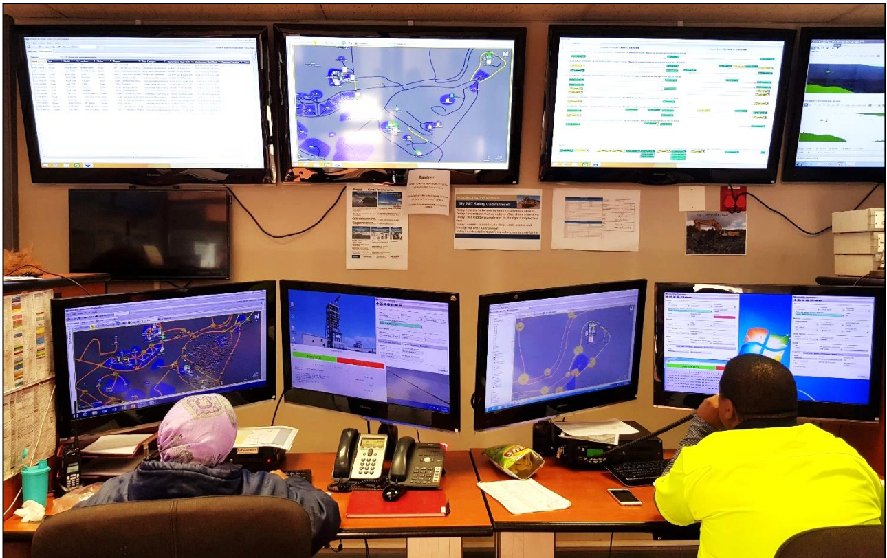
Figure 9: A view of the mines Dispatch control room.
