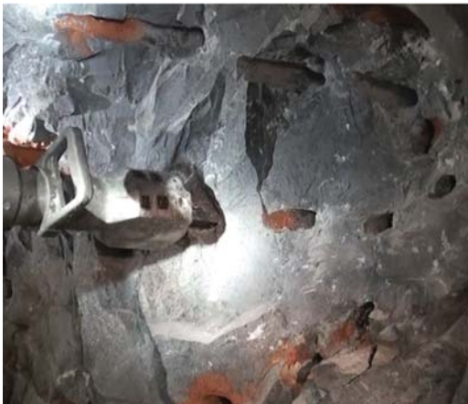
Figure 10—Free face slicing with visible drill barrels parallel to the free face
