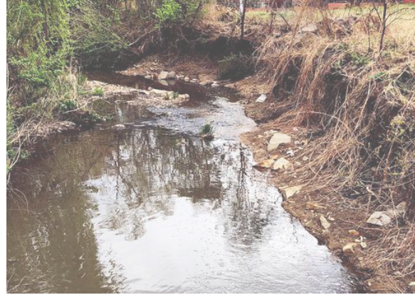
Fig. 1.1 Erosion alongside natural river (Pinterest, 2018)
