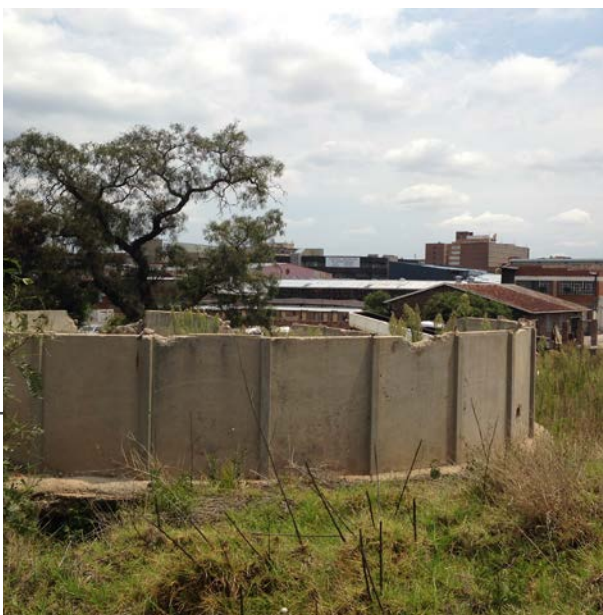
Fig. 1.10 Storage tank (Author:2018)
