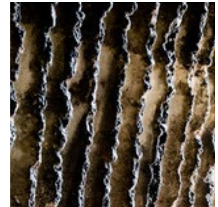
Figure 7.17: Concrete wall burnt (ArchDaily, 2016)
