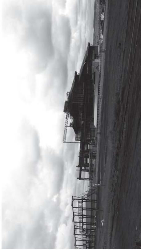
Figure 9. Site photo of static voids that are the result of demolition. (Author, 2018)
