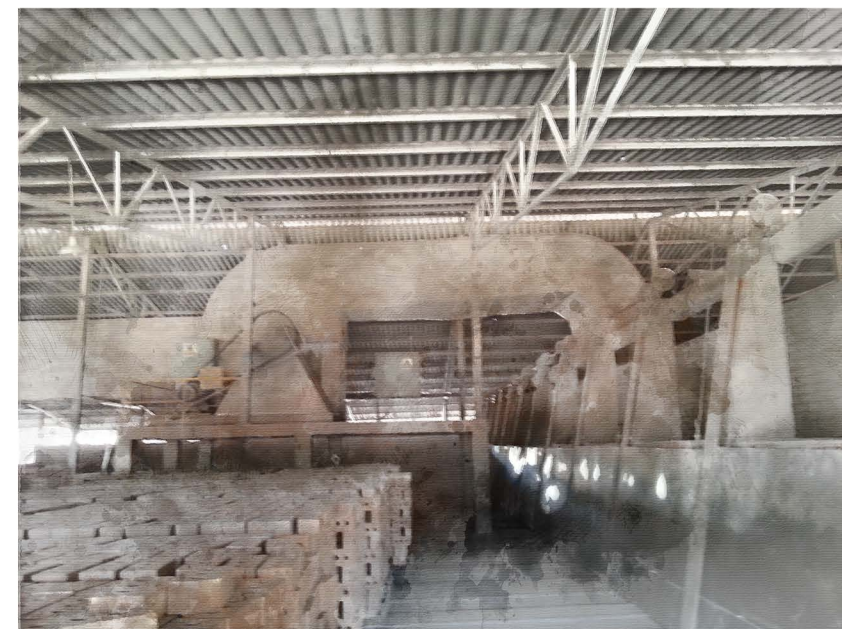
ACTIVE BRICK DRYING TRACKS
