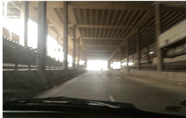
Figure 3.33 - Extension to the mall creating a tunnel road underneath it. The tunnel is aesthetically unpleasing and occasionally floods (Author, 2018).
