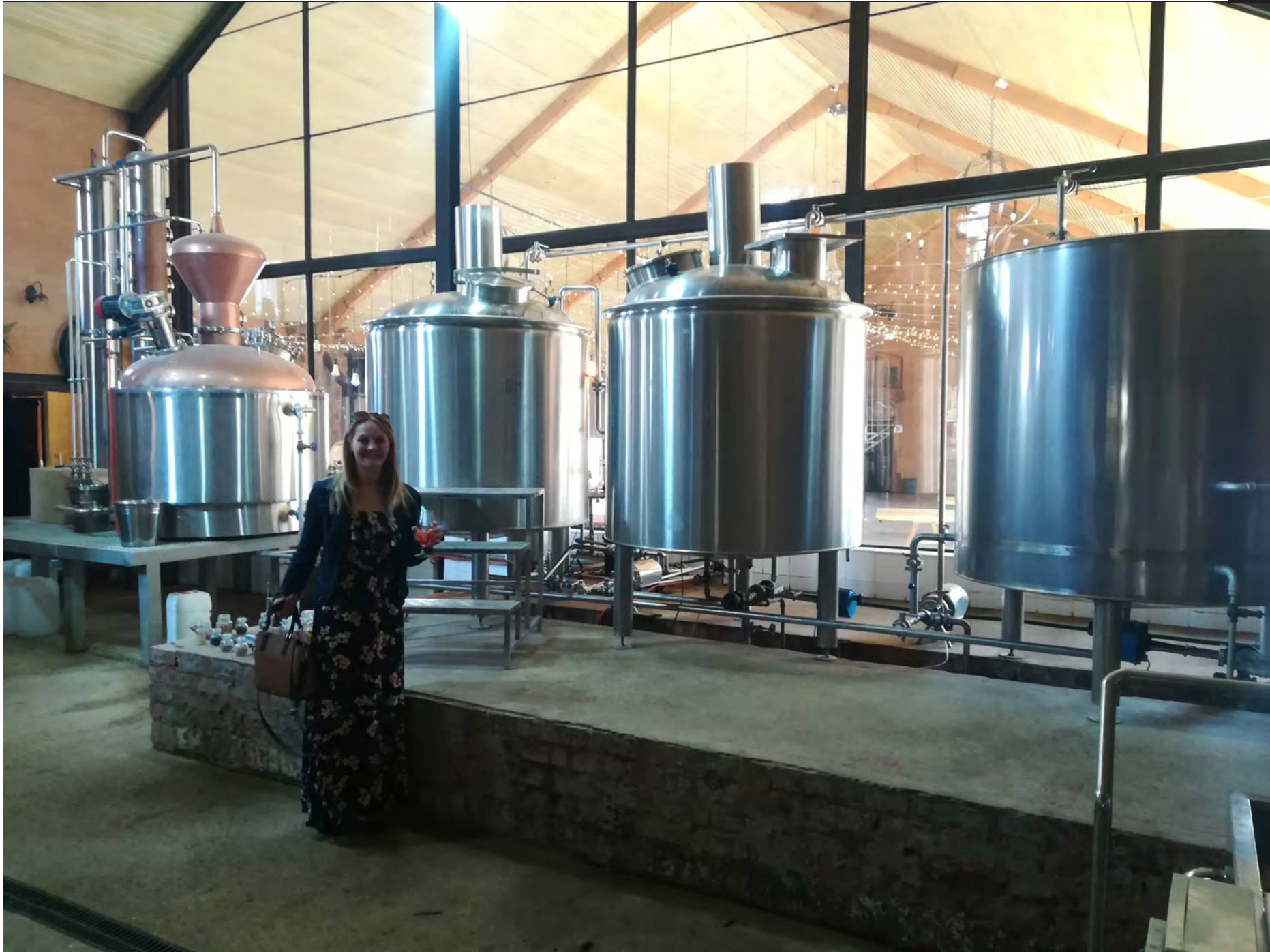
Figure 5.36 - Photography hinting at the placement and general layout of the stills, boilers, mashing tuns, and fermentation vats. Note that the vats are placed on a concrete plinth to distribute the weight across the floor (Author, 2018). © University of Pretoria
