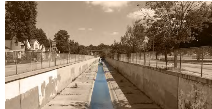
Figure 1.4 - (Garrett and Garrett, 2018). Channelized urban rivers that serves as the epitome of the human need to control nature. Ecosystems were removed and replaced by concrete channels that undermines the potential that rivers can have within the urban construct.
