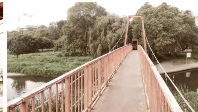
Figure 3.53 - Pedestrian suspension bridge indicating the public park in the background, overgrown by vegetation due to a lack of maintenance (Author, 2018).
