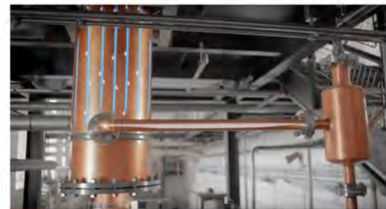
5 Condenser and Spirit Safe: Condensation and Storage Process
