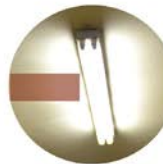
Interior Ceiling Fixture: Fluorescent tube have been placed in every room.
