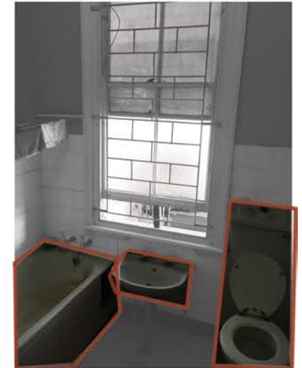
Bathroom 1: The sanitary ware has been replaced. The wall and floor tiles remain the original.
