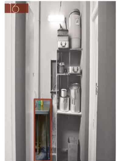
Kitchen 5: The kitchen original cupboards have been removed and replaces with stainless steel work tops. The plumbing has been altered to support the change.
