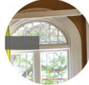
Window Frames & Pelmet: The beading around the windows are original, including the pelmet..
