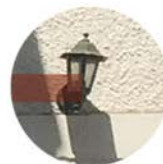
Exterior Wall Fixture: Outdoor wall lights were installed at a later stage.
