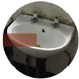
Basins: The basins through the house have been replaced including the mixers.
