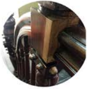
Balustrade 1: The staircase has been altered. Parts of the balustrade is the original kiat turned timber.
