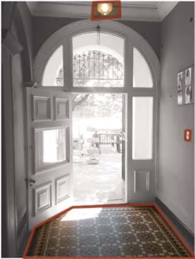
Entrance: The floor tiles, door and light are original. The original copper light switches were stolen and replaced with plastic fittings.
