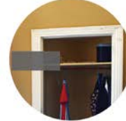
Door Frames: The beading around the doors are original, including the pelmet..
