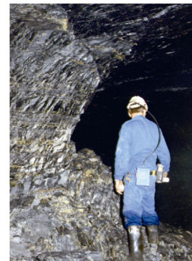
Fig. 9. Scaling of a coal pillar in the Vaal Basin in South Africa [50].
