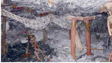
Fig. 1. An example of minor damage caused by seismicity in a deep gold mine in South Africa.
