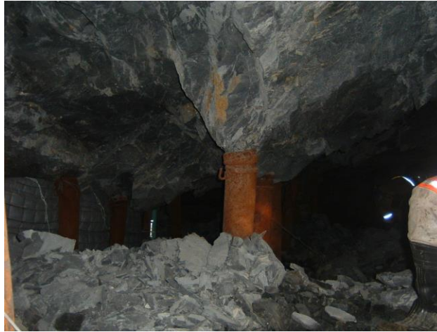
Fig. 13. A photograph illustrating the fallout between adjacent rows of elongates following a seismic event. Retaining support elements between the rows of elongates are required to prevent this fallout (photograph D.F. Malan).
