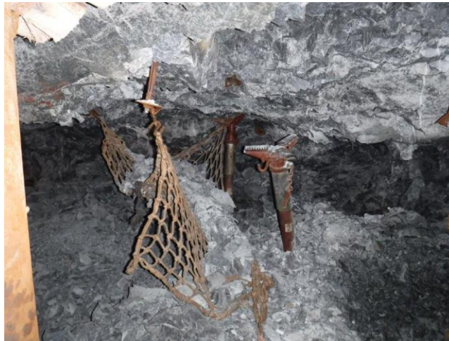
Fig. 14. Example of the failure of a weak retaining element (a removable net) during a rockburst. These nets are typically attached to the bolts and the removable steel props (photograph J.C. Esterhuyse).
