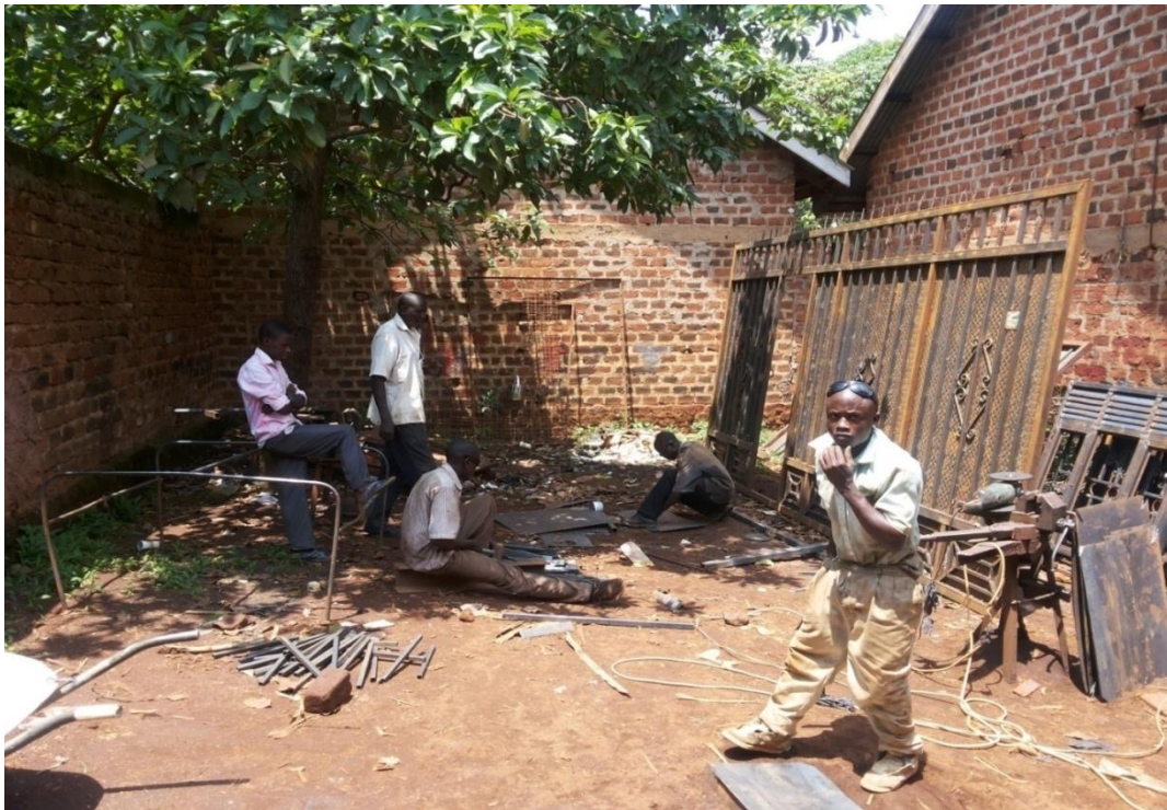
Figure 3: Lule's employees finishing off their work at the workshop. Photo by candidate
