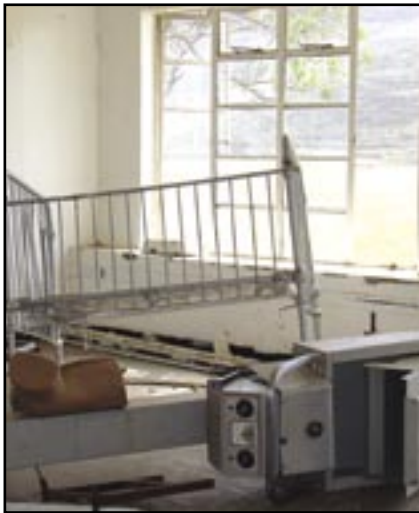
One of the wards in the derelict Semonkong Hospital.
