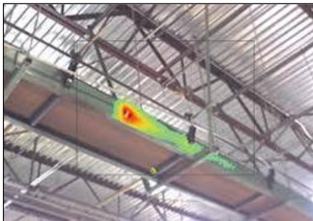
Figure 1.18: Thermal image overlay of elevated conveyor (FLUKE, 2015)
