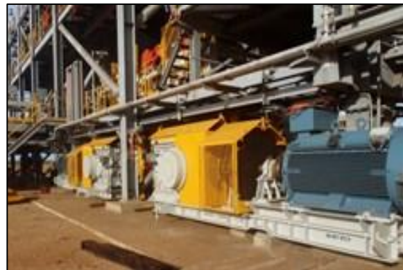
Figure 1.6: CX Conveyor Drive unit installed on site (David Brown, n.d.)
