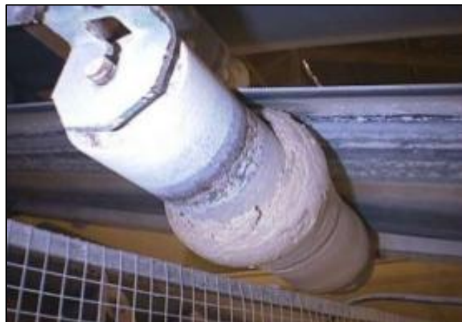
Figure 1.14: Material build-up and visible belt damage (Kinder, 2013)
