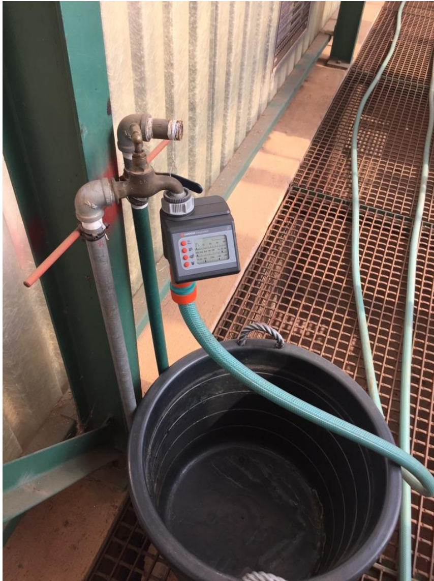
Figure 56 - Irrigation control unit, greenhouse study
