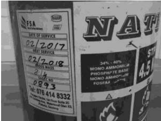
FIGURE 3. Close-up view of the label of the fire extinguisher recovered fully. 8
