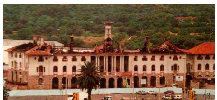
Figure 43. The Burnt out shell of the Station Building, where fortunately only the ground floor and roof levels were completely destroyed. This resulted in upgrades and maintenance that was long overdue (Intersite: 2001).
