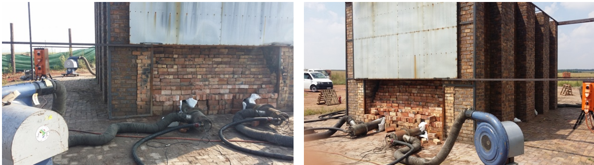
Figure 86: Model kiln firing set up using propane gas as external fuel from the northern end (left) and southern end (right) of the model kiln – Propane gas is fed from storage vessels through evaporators to four individual burners that deliver a 3 m flame length into the vents (vent openings are sealed off with mineral wool)
