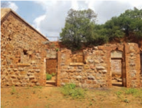
Fig. 63c. Fort rooms detreated walls (Author 2017).
