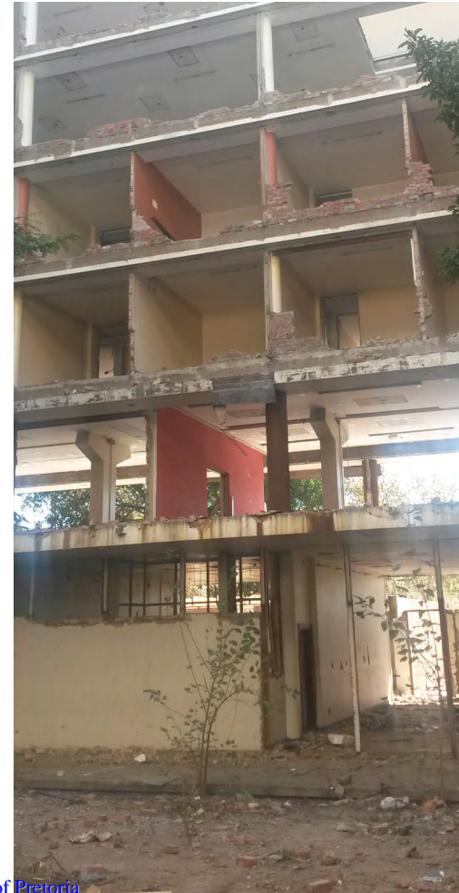
Figure 32: C-block - Damage to southern façade.
