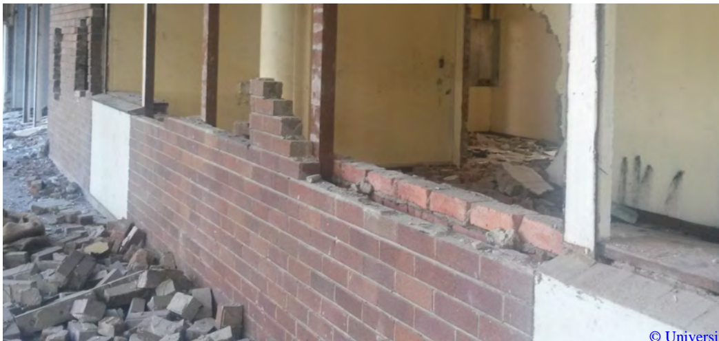
Figure 28: C-block - Damage to southern facade.
