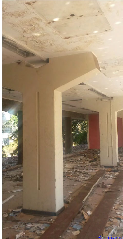
Figure 31: C-block - Damage to first floor.
