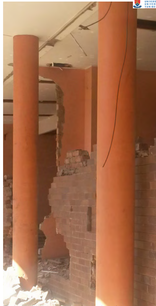
Figure 27: A-block - damage to northern facade.
