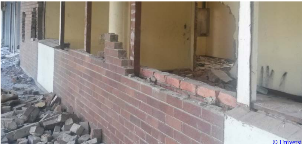
Figure 28: C-block - Damage to southern facade.
