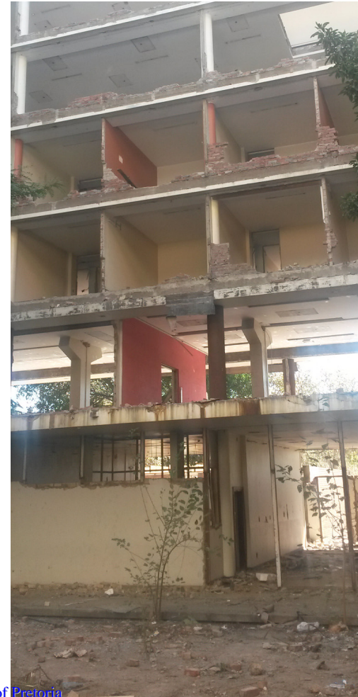
Figure 32: C-block - Damage to southern façade.
