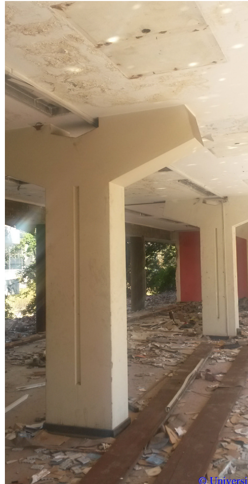
Figure 31: C-block - Damage to first floor.
