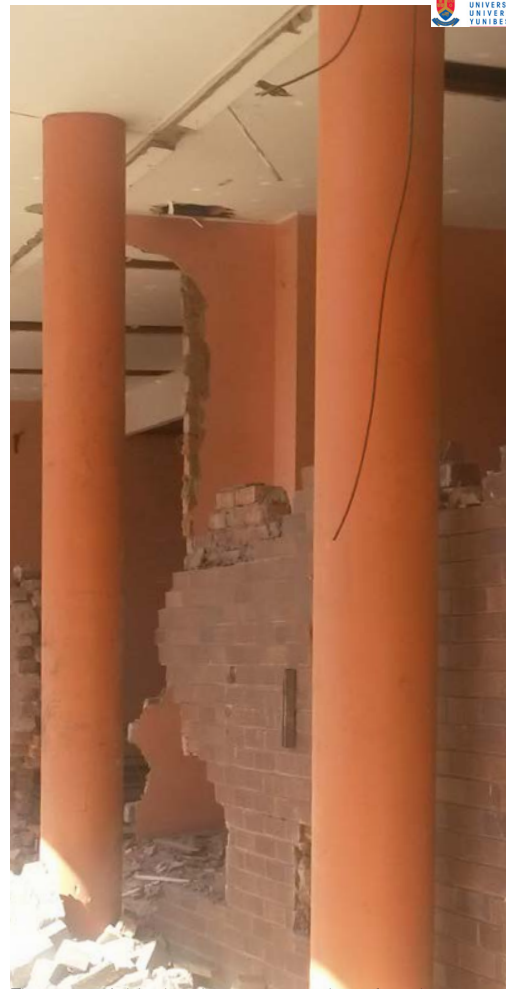
Figure 27: A-block - damage to northern facade.
