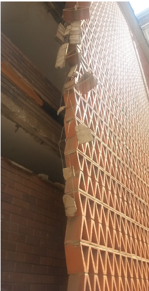
Figure 26: B-block - Damage to briti tiles.
