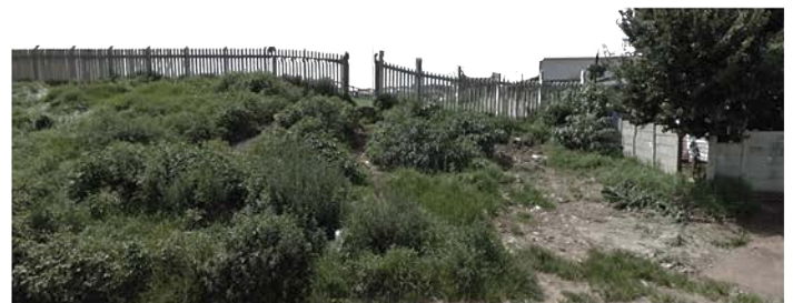
Fig.6.5: Illustration showing eroded slopes in Du Plessis Street (Author, 2017)
