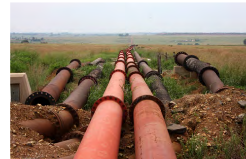
FIG 39 : (Above) “Over one thousand kilometers of pipeline connect the historic mine dumps, gold processing plants and new super dumps in a vast network that covers the region. Under 45 bars of pressure, the pipe network delivers new gold slurry to processing plants and reprocessed waste to super dumps. Roughly 30 percent of the water used in this cycle is lost to evaporation or seepage” (Tang, Watkins, 2011)
