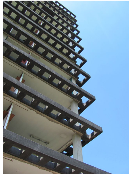
Figure 114 - View of brise soleil from ground level with framing pattern (by Author)
