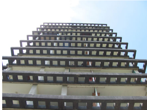
Figure 39 - Northern façade with missing cladding (by Author)
