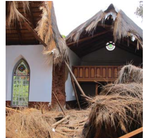
Fig.2.15 Photo of the church's collapsed thatch roof (Author, 2017)
