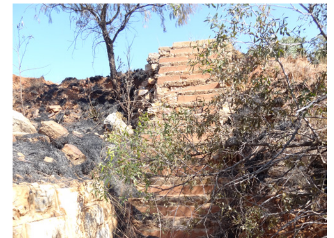
Figure 7.177 Deterioration of the existing stairs
