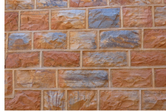
Figures 3.20a A construction of the local stone, detailed with a cement finish, used to build the majority of the fort
