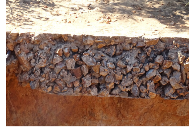
Figures 3.20b Erosion of concrete to expose large stone aggregate
