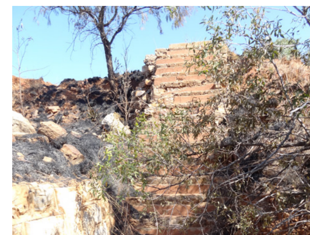
Figure 7.177 Deterioration of the existing stairs
