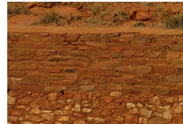
Figures 3.20c A structured construction of the local stone, used to build supporting walls
