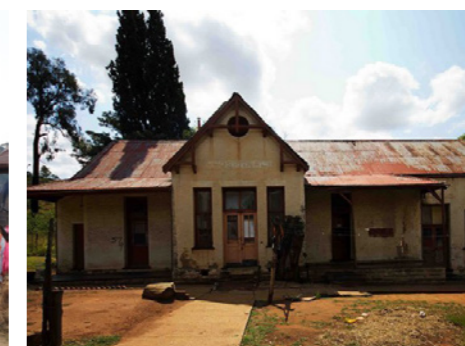
Figures 3.9e Dilapidated structure
