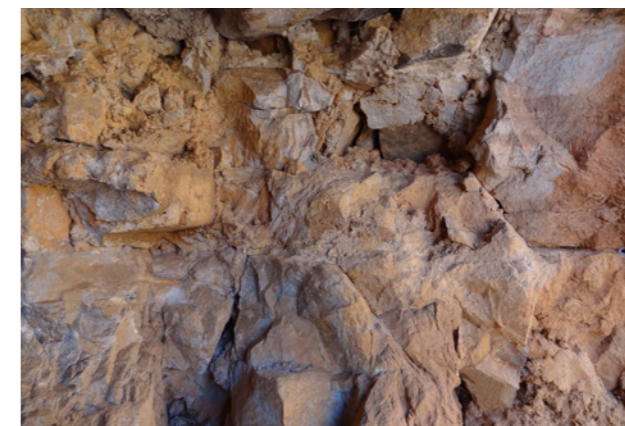
Figures 3.20e A combination of the natural stone and cement, used to retain earth
