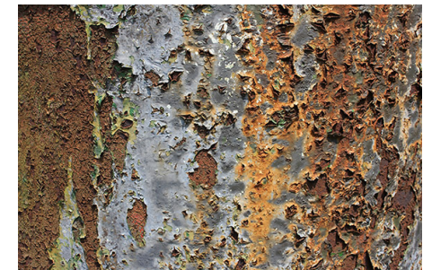
Rusted painted steel
