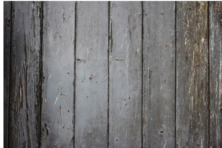
Weathered timber doors
