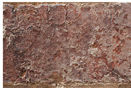
Weathered clay bricks
