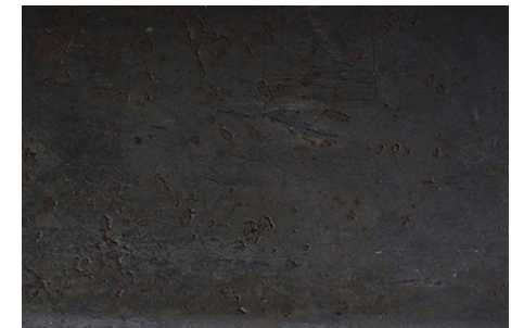
Weathered painted steel
