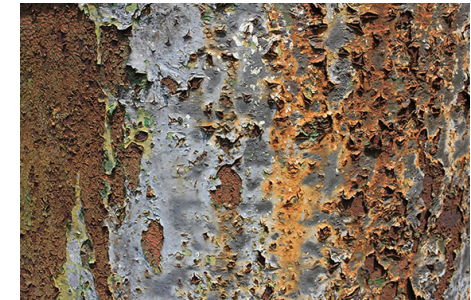
Rusted painted steel
