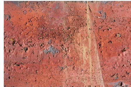
Rusted painted steel
