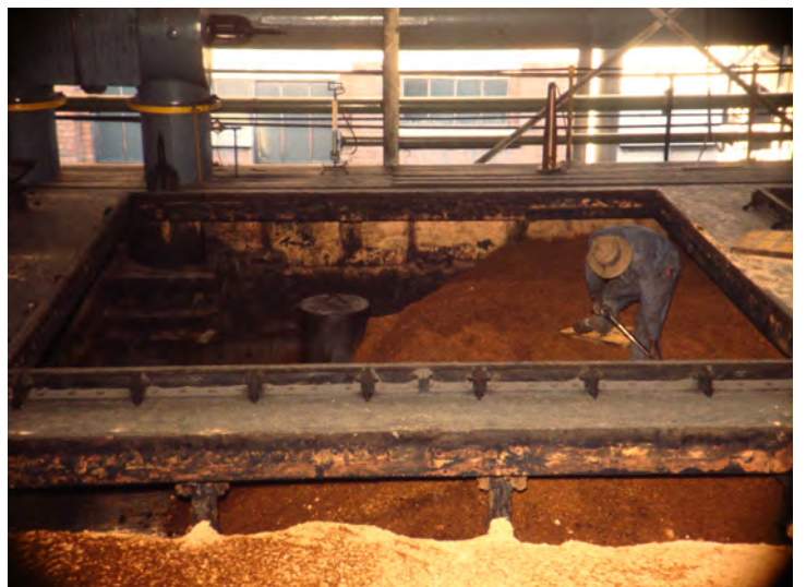
Figure 84 Purification box inside plant (Tsica archives, 2017)
