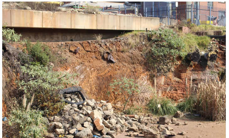
Figure 70 Hole 1 edge condition. Photograph by Author (2017)
