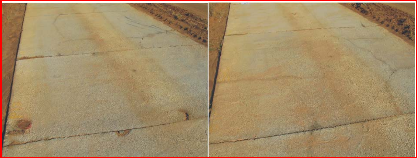
Figure 6: The surface of the plain concrete slabs of section 7
