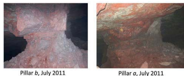
Figure 7—Photographs of pillars a and b during the visit conducted for the stability study (July 2011)
