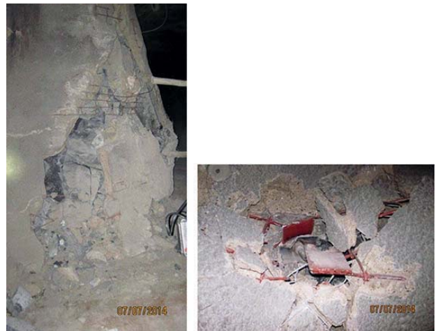
Figure 19—Typical damage to the supported pillars (left) and a roofbolt pulling through the bearing plate as the pillar continued to undergo dilation (right)
