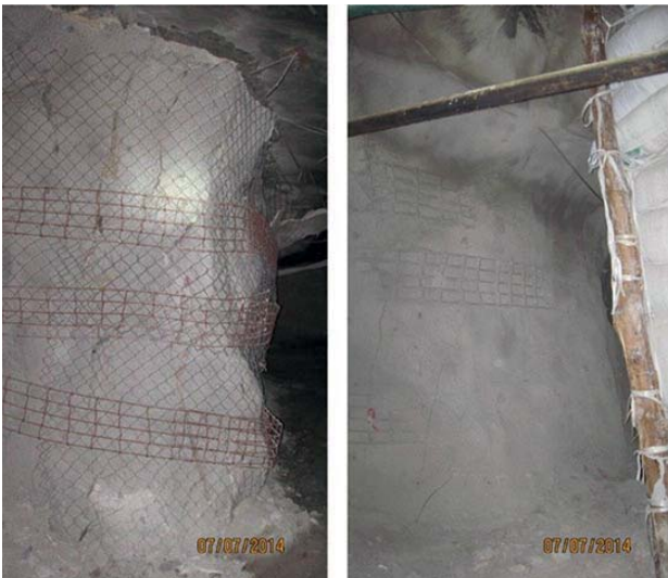
Figure 18—Strapping of the pillars in the mine shown in Figure 17. The strapping consisted of two layers of shotcrete, mesh, and steel straps
