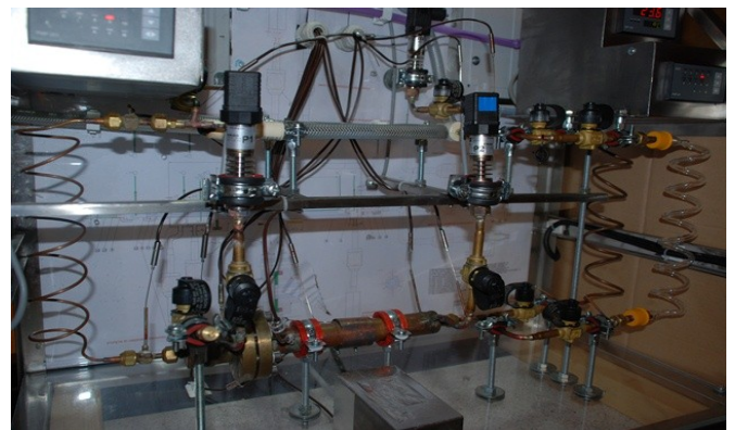
Figure 5 View of the experimental facility without necessary insulation of evaporator, vapour and liquid lines.
