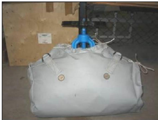
Figure 77: Example of valve insulation (Adapted from McComb 2013)
