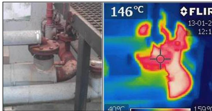
Figure 76: Uninsulated steam lines (Adapted from McComb 2013)
