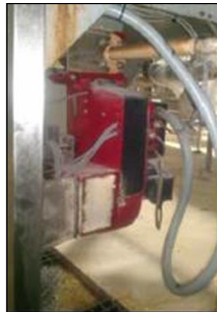
Figure 75: Burner intake (Adapted from McComb 2013)
