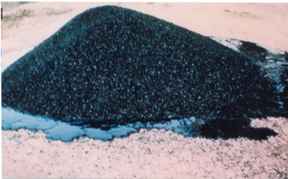
Picture 1. “Drain Down” Due to Lack of Fibers.
