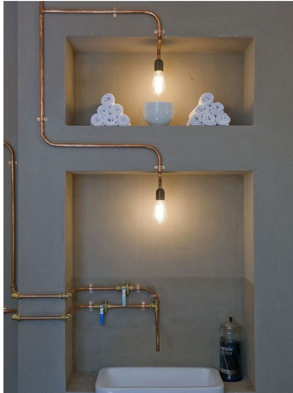
Fig 7.26. Exposed water and electrical conduits (Masquespacio 2016).
