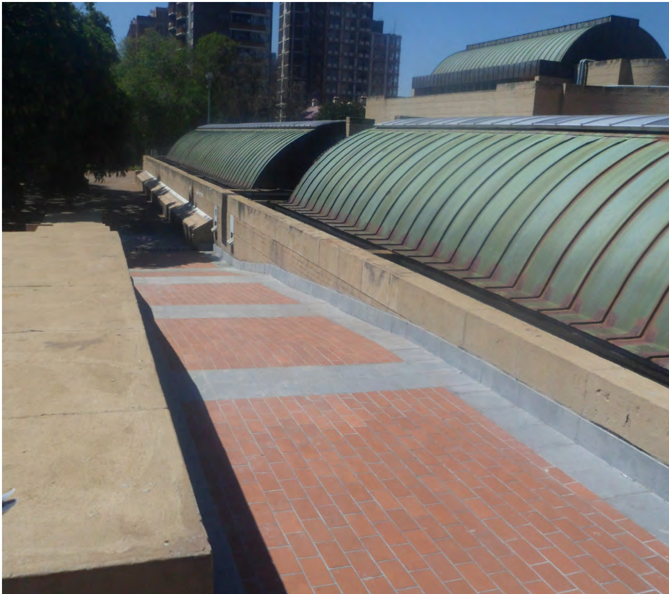
Figure 3.23: Ramps leading onto entrance platform alongside relentless and dead roofs and retaining wall.
